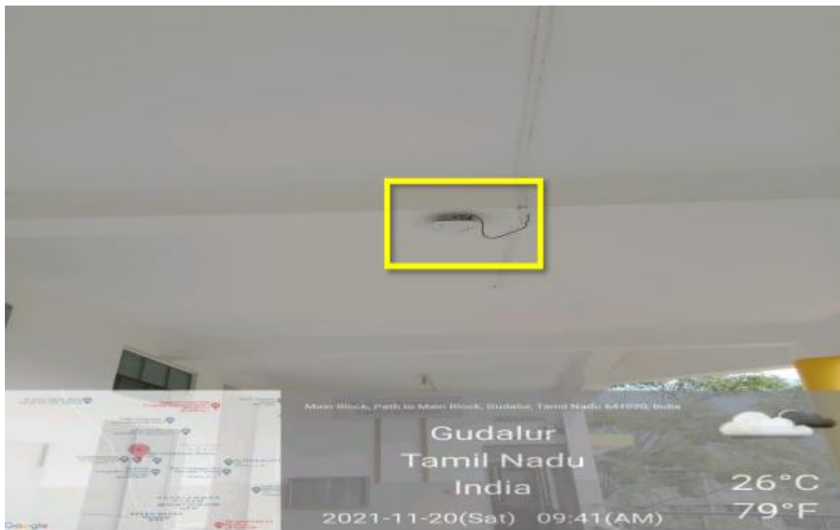
Wi-Fi router in C Block First Floor
