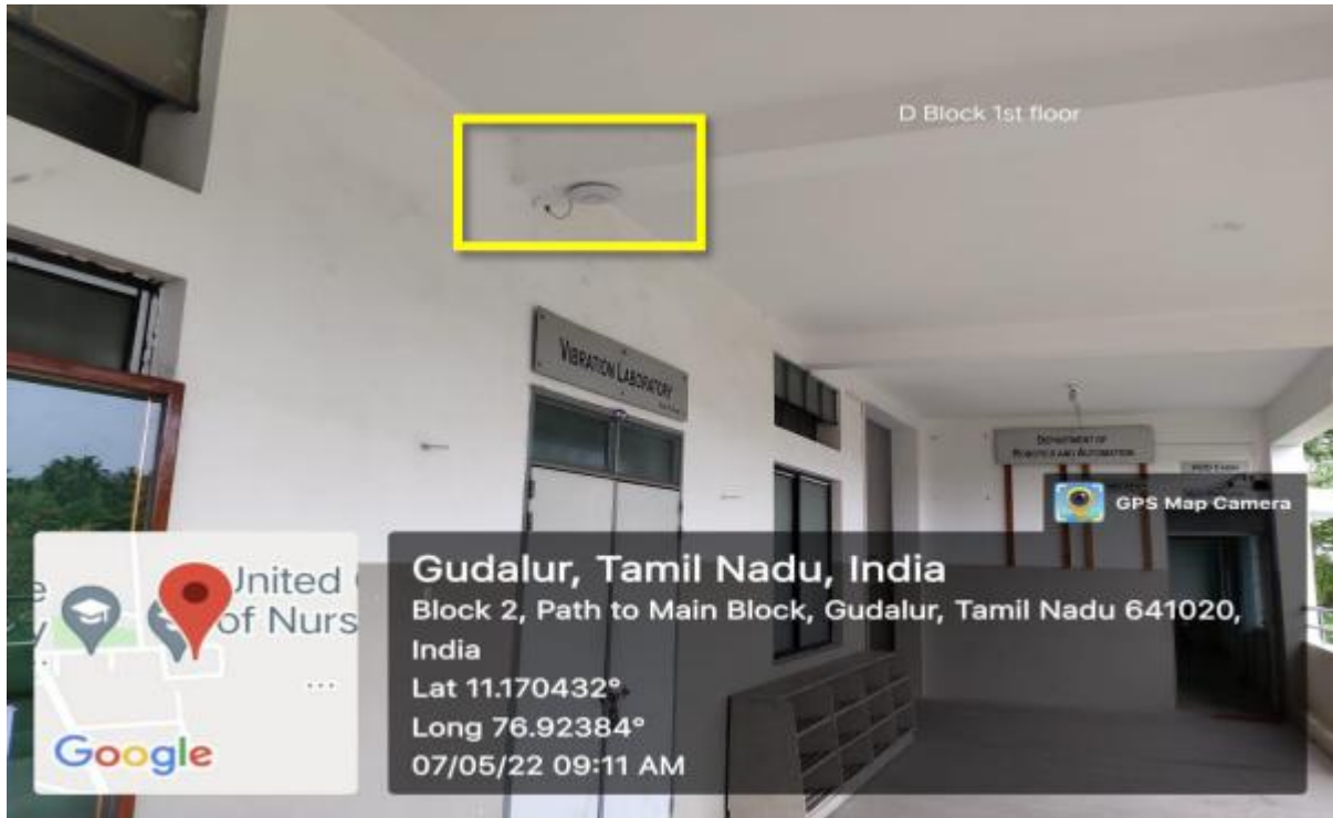
Wi-Fi router in D Block First Floor
