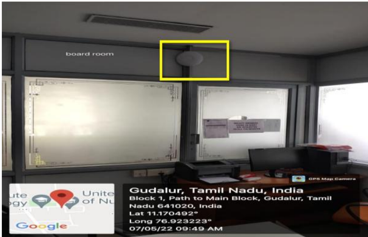
Wi-Fi router B block Board Room
